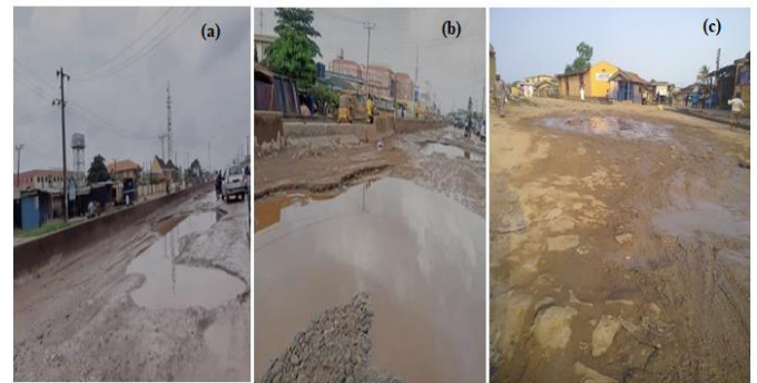
Figure 1: Failed section of Sango-Ota-Idiroko Highway; (b) Abandoned section of Sango-Ota-Idiroko Highway; (c) Dilapidated inner road off Sango-Ota-Idiroko Highway.
