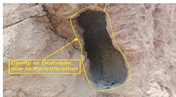
Figure 8: Karstic cavity in dolomite of Drinjal Formation.
