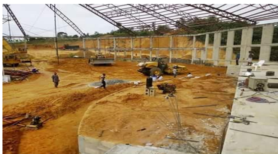
Figure 1: The collapse Reigners Bible Church structures
